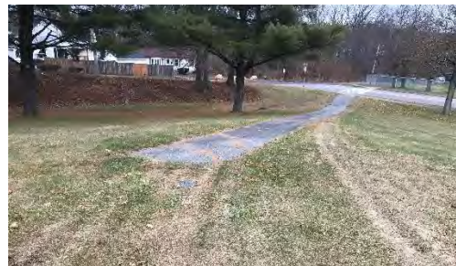
Cracked bit. concrete pathway
