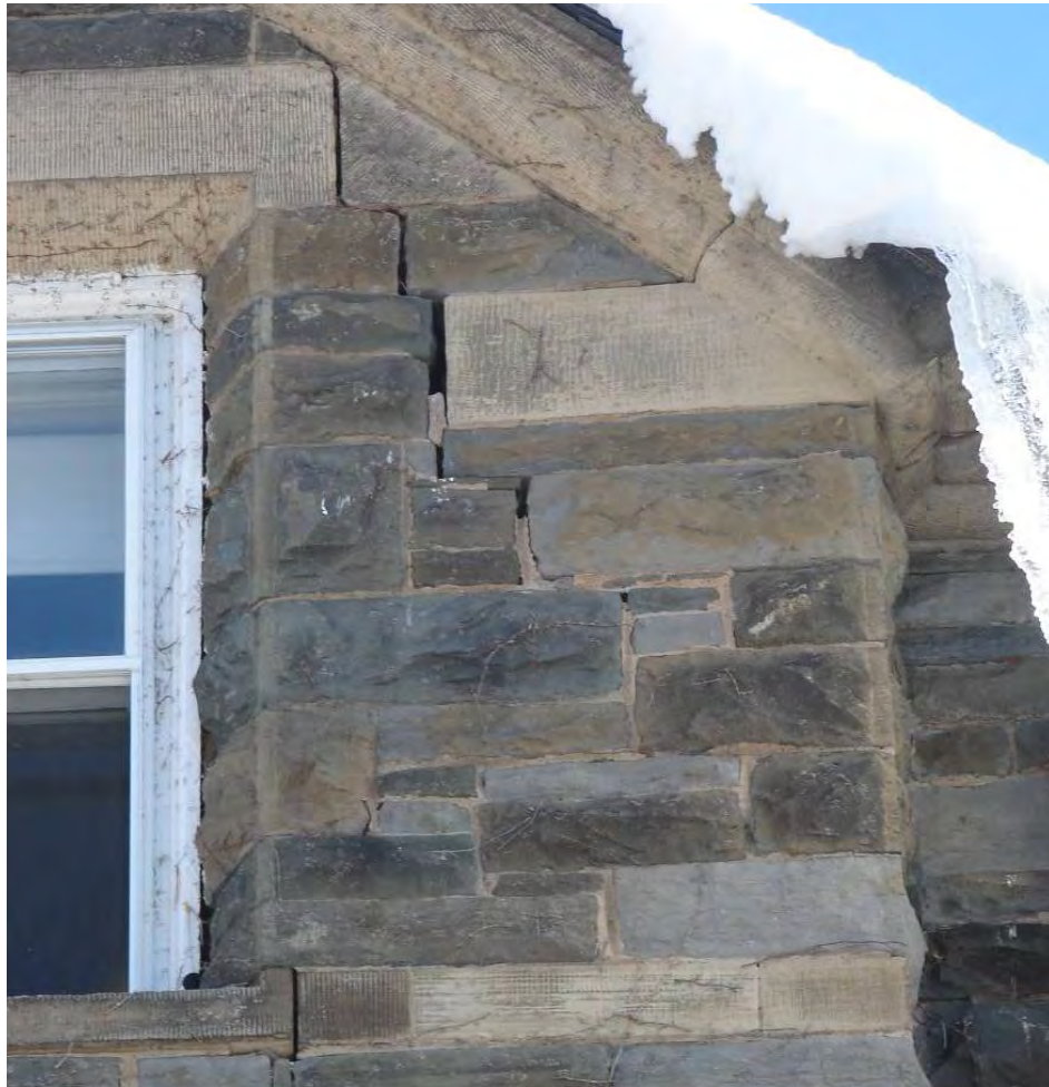
Open joints in a stone masonry wall and related cast stone features.
