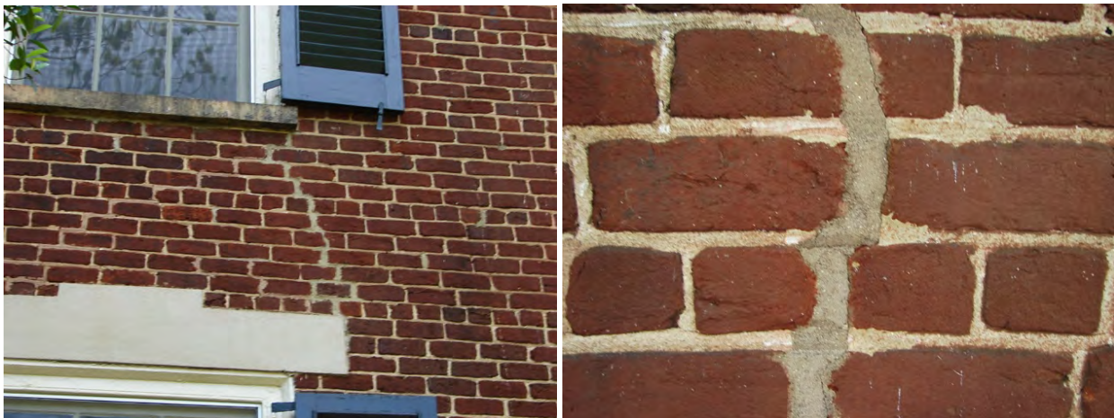
Cracking is often sign of a structural issue that needs to be addressed. In both these examples, cracking occurred not only along the joint line but also through the bricks themselves. Both of these were improperly repaired (see Pointing and Mortar below).
