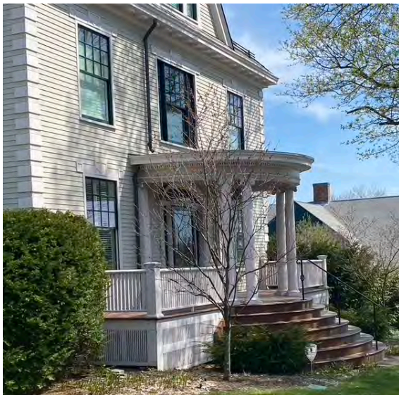
The gutter above was positioned near the center of the front elevation so not to distract from the building’s elaborate wood corner detailing.
