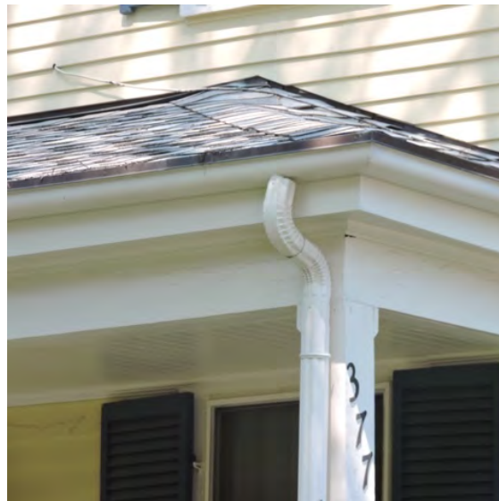
The porch roof above has built-in wood gutters lined with metal, important historic features that have been preserved and maintained.
