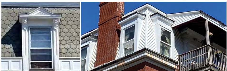
The mansard window on the left is preserved and protected. The mansard, windows, and window detailing on the right have been inappropriately replaced.
