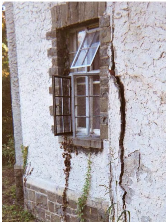
Stucco finish of a Tudor style building delaminating from the wall to which it was applied
