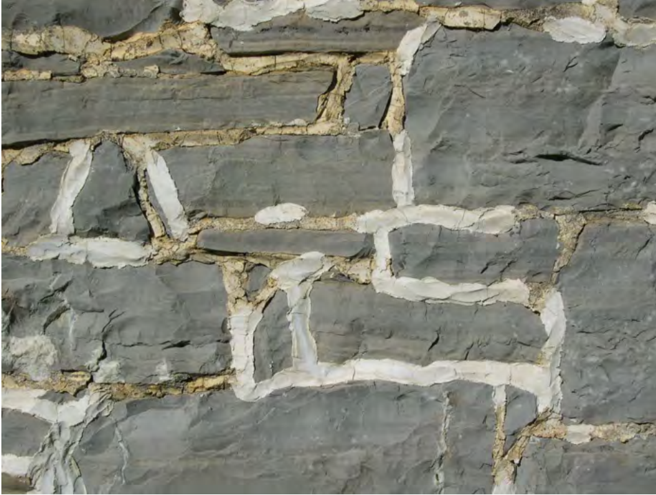
Improperly repaired stone pointing – similar to the mortar and pointing issues for brick walls discussed in the previous section of this chapter.
