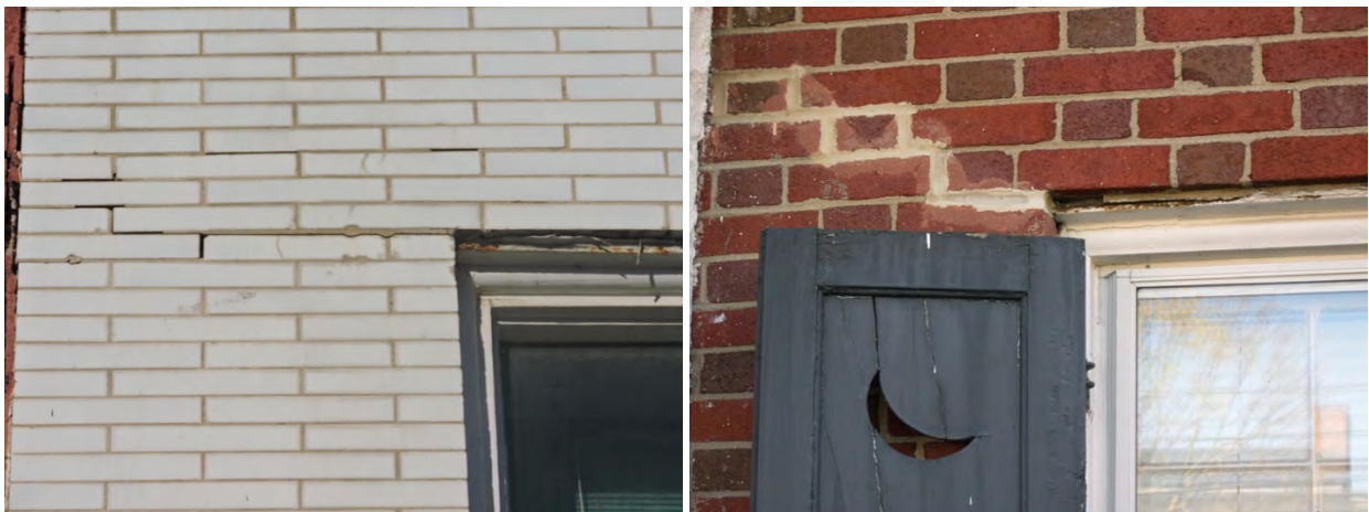
Rusting steel lintels have caused jacking in both of the examples above. The resulting crack in the photo at the right was improperly repaired.
