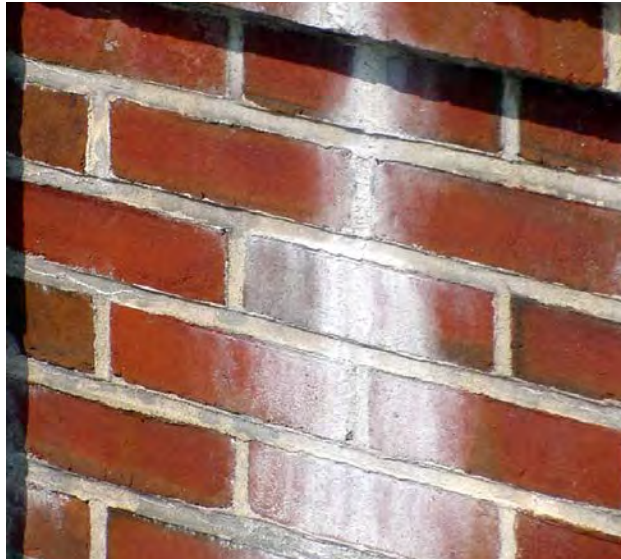
The white stain on the brickwork above is efflorescence.
