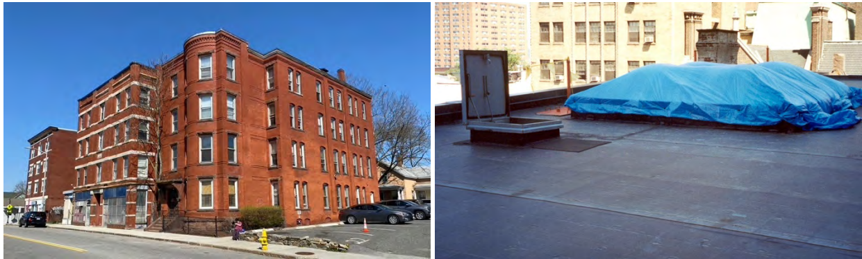
Membrane roofing is appropriate for nearly flat roofs that are not visible from the street.
