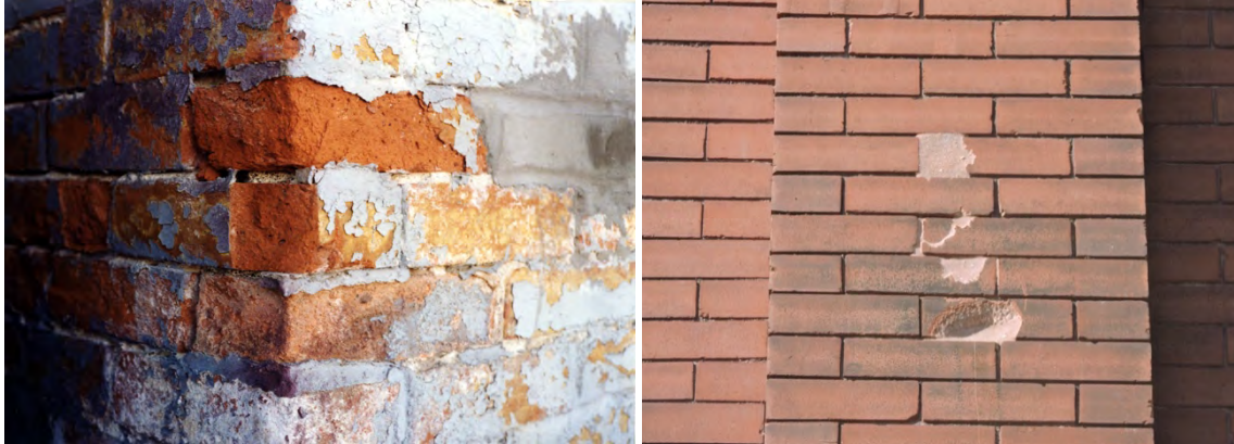
Spalling has occurred in both photos above, where freezing of water within the brick has caused the surface of the brick to flake off.
