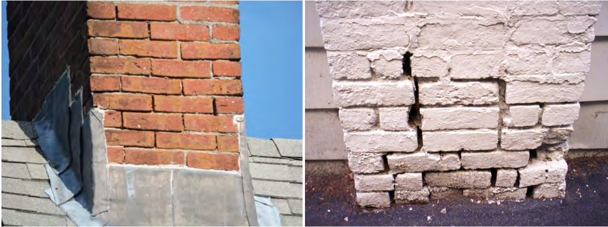
Open joints in the chimney top (left) and chimney base (right) allow water to enter the wall, erode mortar, and cause damage when it freezes.
